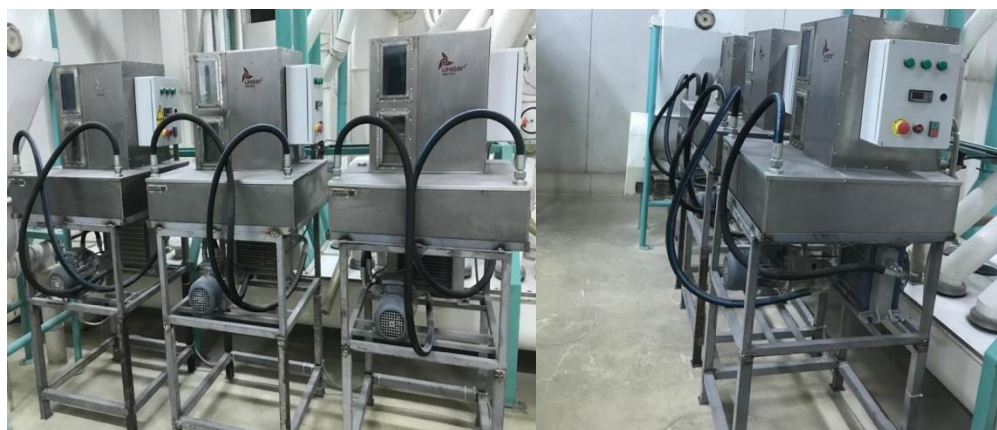
Fig 1 UNISER ozone generator
